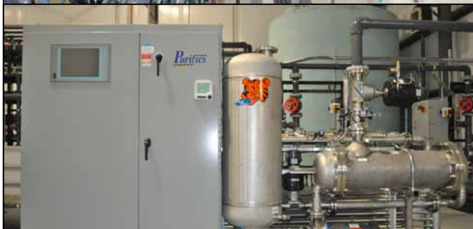
(Fig.3a - above) Landfill Area treatment system (Fig.3b - below) UV Oxidation unit destroys contamination
