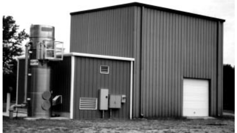
The new carbon treatment facility at the Clapp and Whitcomb wells is used to remove color from the water.
