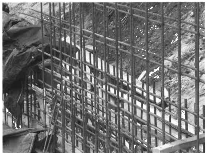
The Kennedy-Marshall Treatment Plant required much steel rebar reinforcement. The skyrocketing cost of steel is one of the reasons construction costs have escalated.
