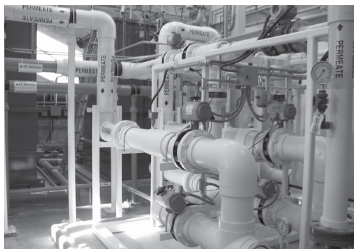
Inside the recently completed North Acton Water Treatment Plant. Filtered water is pumped through these pipes for disinfection and distribution to our customers.
