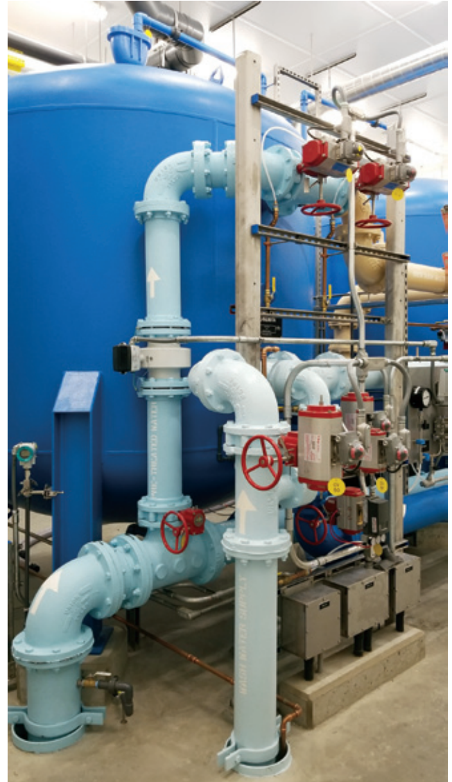
Newly installed pressure-filtration vessels in the Central Acton Water Treatment Plant located off of Post Office Square.
